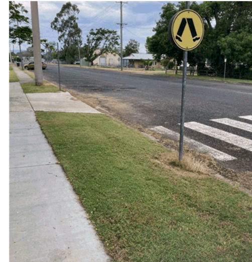
Queen St - Missing kerb ramp and path connections at school
