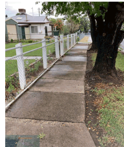
Path damaged by tree roots, Rutherford St
