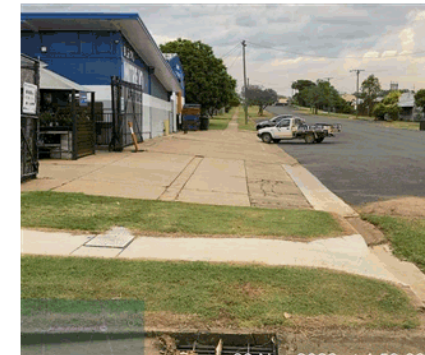
Missing kerb ramp and path at Stuart Russell St
