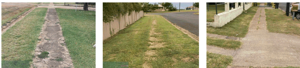
Examples of paths in poor to very poor condition, impacting on use by wheelchairs, prams etc
