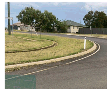
Missing kerb ramp/s – Leichardt St / Mahoney St
