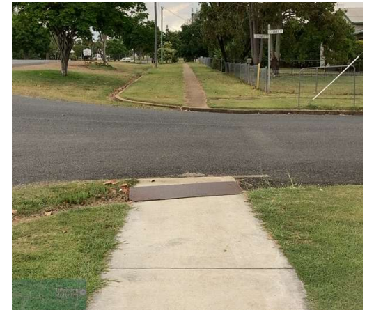
Missing kerb ramp – Leichhardt St/Perry St
