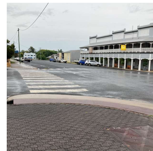
Missing warning signage at crossings in Lister St
