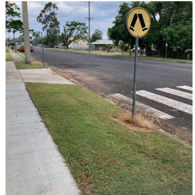
Queen St - Missing kerb ramp and path connections at school
