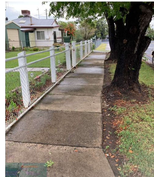
Path damaged by tree roots, Rutherford St
