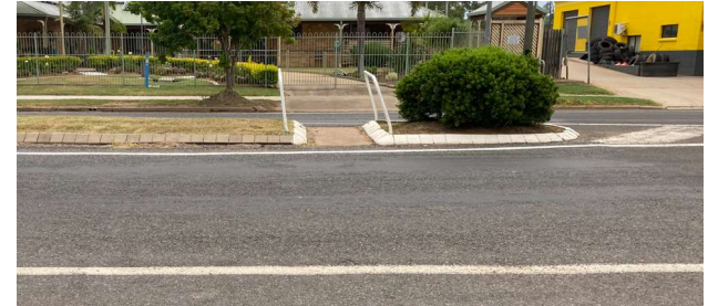
Capper St crossing point - shrub potentially obscures pedestrians
