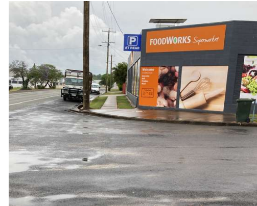
Missing kerb ramps, Lister St
