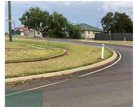
Missing kerb ramp/s – Leichhardt St / Mahoney St
