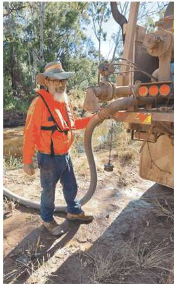
Above: Dulong Road shoulder repairs: water truck driver complying with WHS whilst filling water truck.
