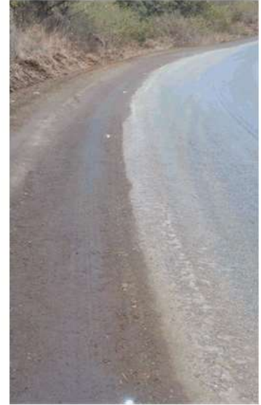
Above: Biggenden Mines Road shoulder repair; finished and marked out for bitumen seal.
