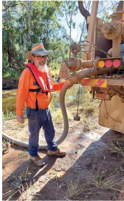
Above: Durong Road shoulder repairs: water truck driver complying with WHS whilst filling water truck.
