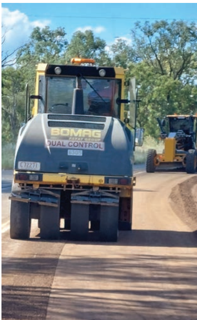
Above: Mount Perry Road stabilisation: Multi tyre roller in front of grader doing the final trim, steel flat drum roller.
